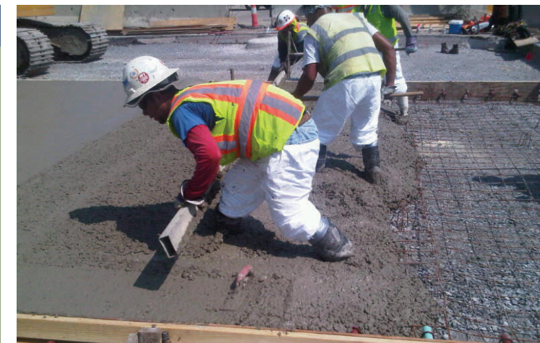
7755 Dwyer Road - Milestone in Sight! Paving of Downman Road; Scheduled to re-open after two years of construction on the multi-phase box culvert.
